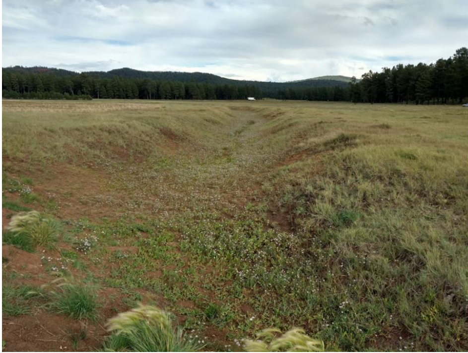
Appendix Figure C3: Unrestored trench in the southeast portion of the site. (September 13 th , 2016)
